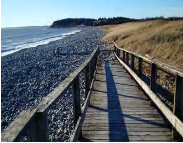
Figure 10: Impacts to beach access infrastructure from winter storms.
