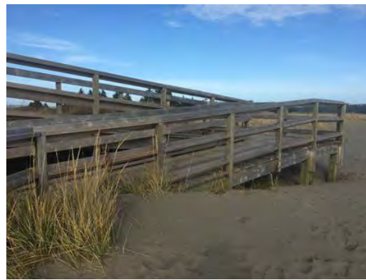
Figure 5: Sand encroaching on boardwalk.
