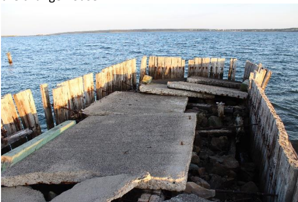
Figure 4: Deteriorating sections of the wharf.
